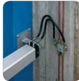
Connection to the 6-way oil pipe block
