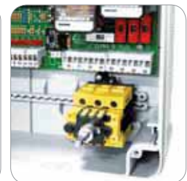
Detail of the disconnecter switch
